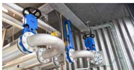
In the digestion tank sludge is recirculated through a heat exchanger.
