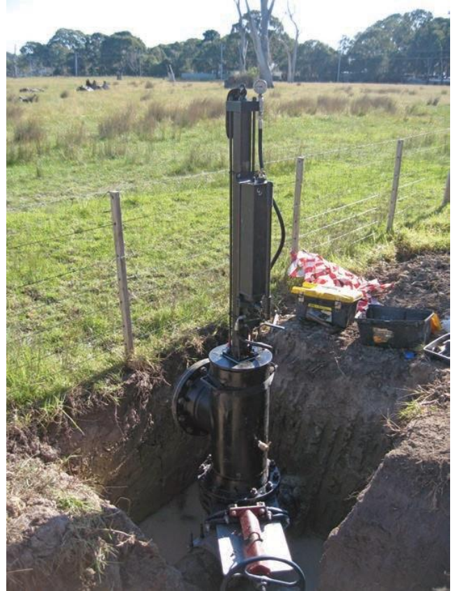
225mm HydraStop at Eagle Point, VIC
