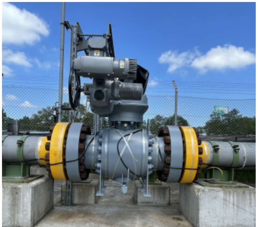
Control ball valve 12" cl1500 as main feed-in and withdrawal control valve for one of the natural gas storage caverns in Etzel (with trace heating without insulation in the installation phase)
